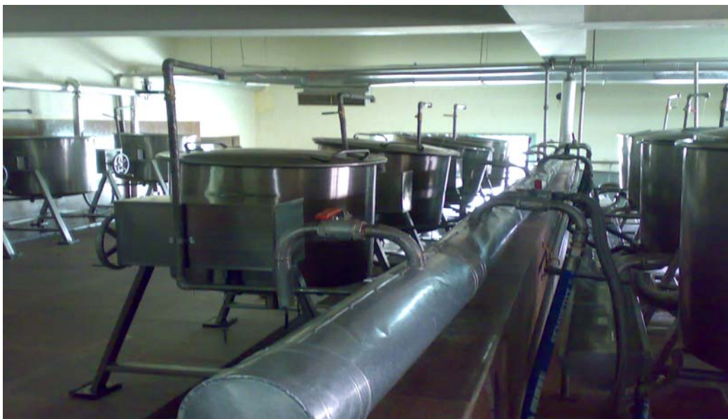
Figure 4.10 : Boilers for Cooking Food at Akshay Patra
